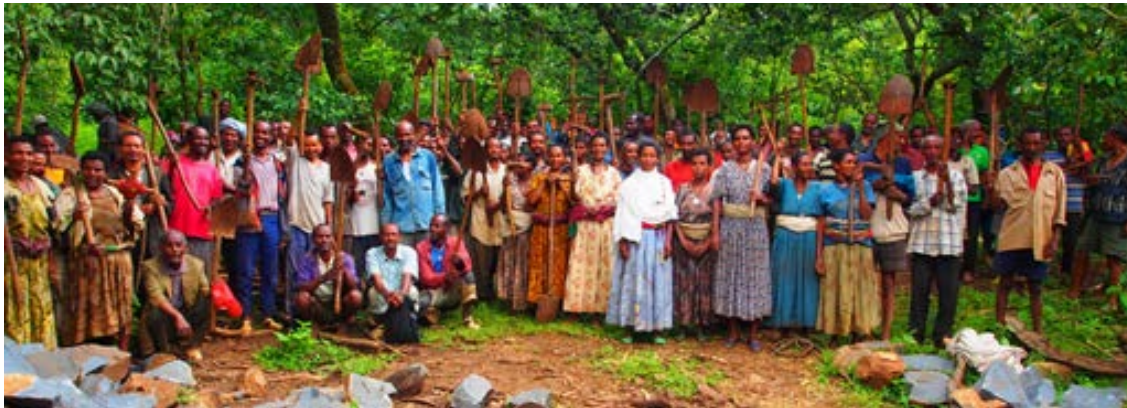
Figure 8.3 Community members in Yiganda, Zegie, near Bahir Dar, wave their spades to reaffirm their commitment to finish excavation on schedule. They are digging trenches for pipelines as their labour contribution to a project to bring water to their village.
