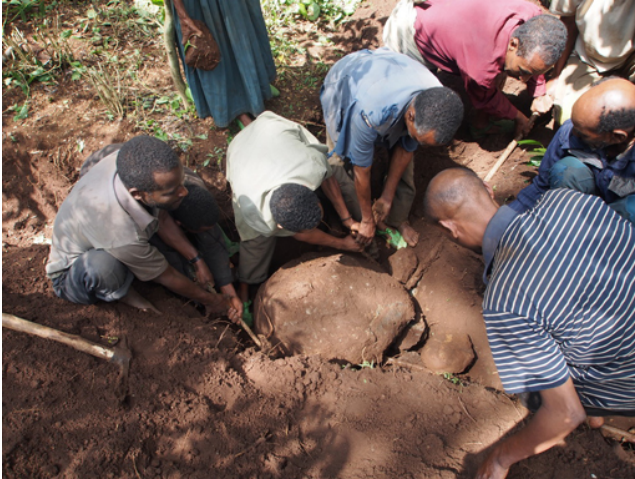
Figure 12.1 Community members in Yiganda, Zegie, near Bahir Dar, excavate trenches as they prepare for water pipes to be laid.
