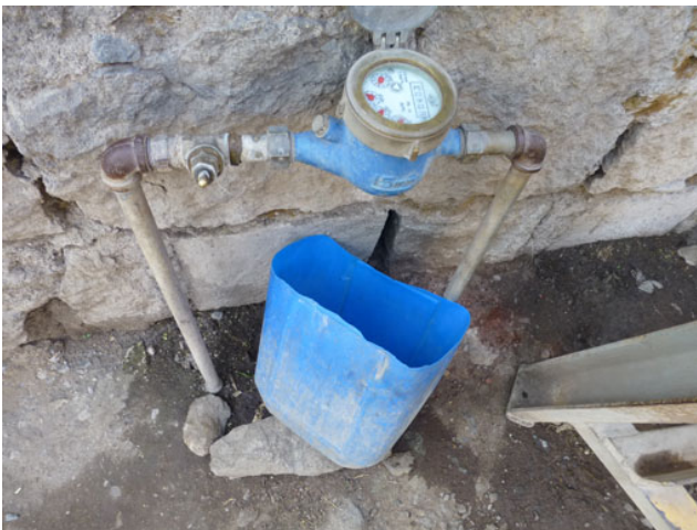
Figure 12.2 A water meter in the yard of a household. Regular meter readings measure the volume of water used and are used to calculate the payment due to the water utility.
