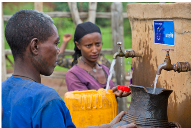
Figure 9.2 A water point in the Amhara region with emblems of UNICEF and the European Union indicating they provided funds for the installation.
