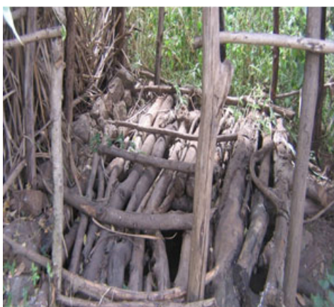
Figure 10.7 An example of an inadequate pit latrines.
