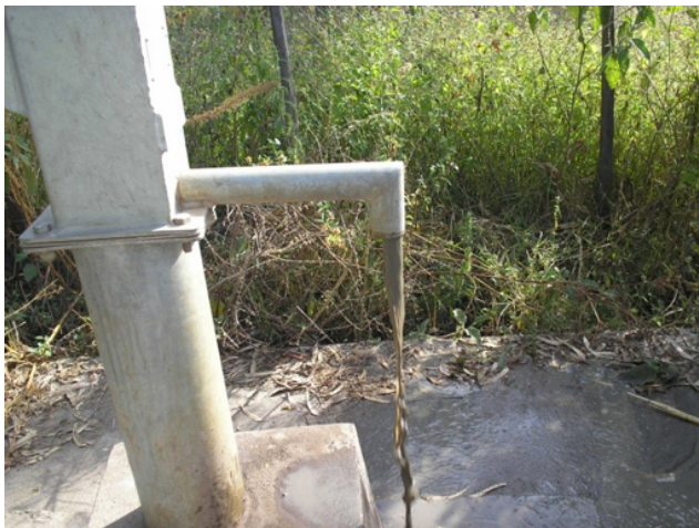
Figure 8.4 Water infiltrated this well in the Shashogo district of the SNNPR during a flooding disaster and now the water is muddy and unusable.
