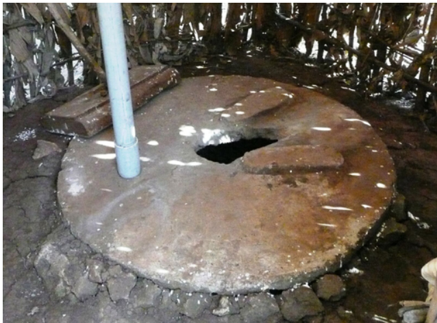
Figure 13.6 It takes time and effort to convince people that building a covered pit latrine like this one will benefit their family’s health and improve the local environment.
