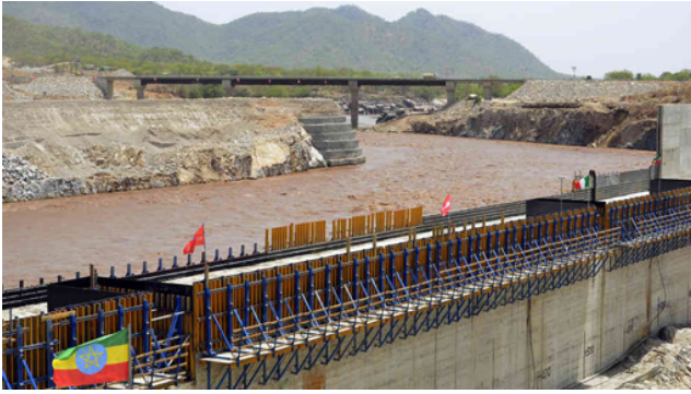
Figure 12.2 The construction site for the Grand Ethiopian Renaissance Dam in northern Ethiopia. When completed, the reservoir will cover an area of 1800 km 2 .
