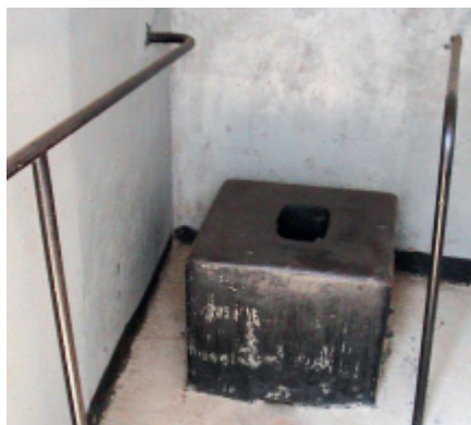
Figure 12.1 Latrine with handrails and raised position to support disabled students.
