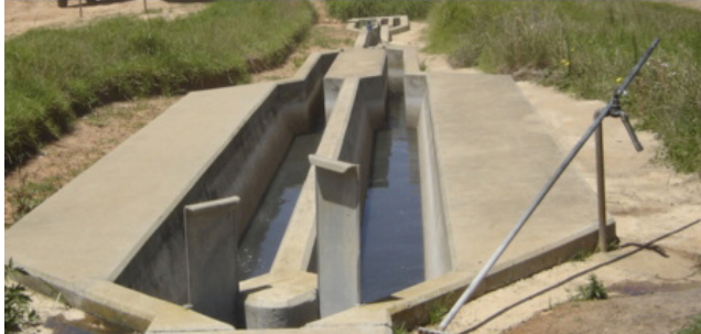
Figure 6.14 A grit channel that slows the rate of flow and allows grit to settle out by gravity.
