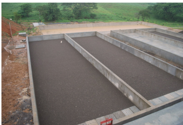
Figure 6.4 Sludge in drying beds.
