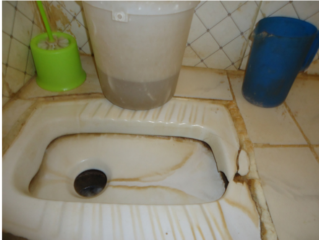
Figure 5.16 A pour-flush toilet. Water is stored in the white bucket and the blue jug is used for pouring water in after use.
