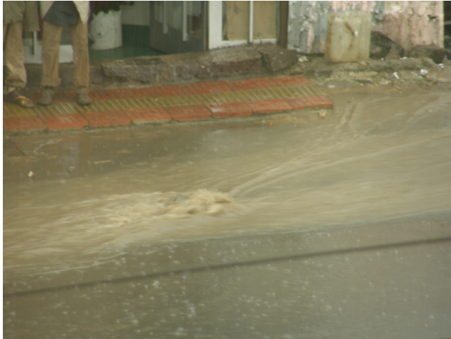
Figure 4.4 Stormwater flow during the rainy season in Ethiopia can sometimes exceed the capacity of the drains.
