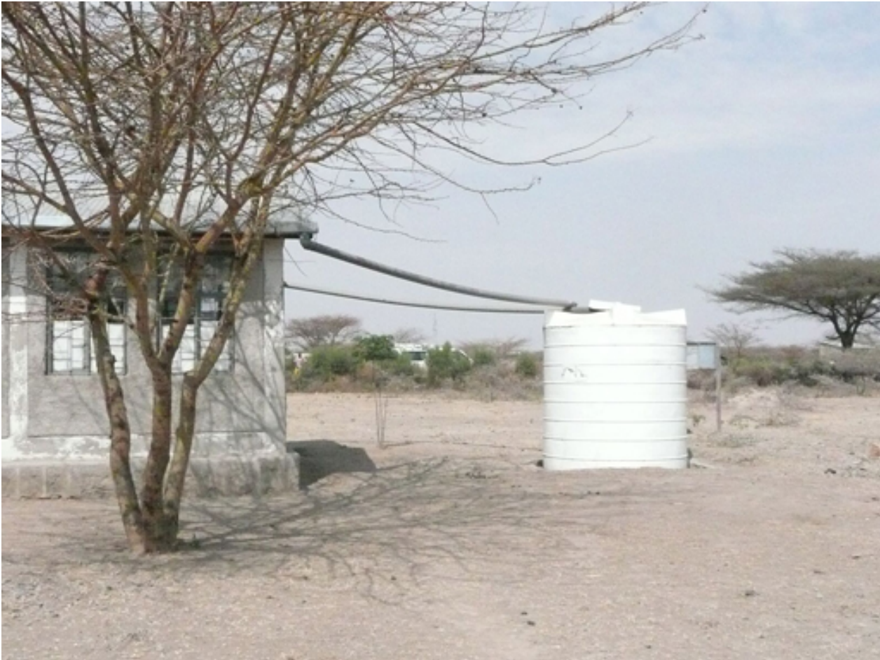
Figure 3.13 Rainwater is collected from the roof of this rural health post and stored in a covered, watertight cistern.
